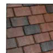
SYNTHETIC SLATE SHINGLE ROOF:
