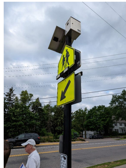
Existing Flashing Beacon at Barry Ave
